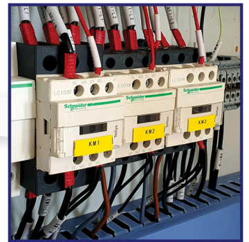
Electrical parts Schneider
